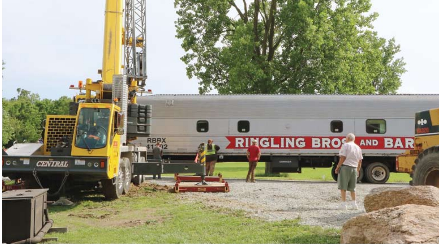
The crane is placing the car on the Miser's section of track beside their pond. Harold Miser is observing on the right.
