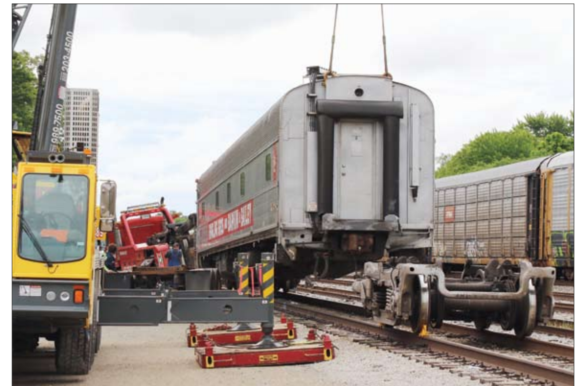
One end of the car is hoisted. At right on the tracks are the set of trucks just removed. The crane on the left has its counter balance extended out so the crane doesn’t tip over. At the other end of the car the tow truck is in place with its stabilizing platform.
