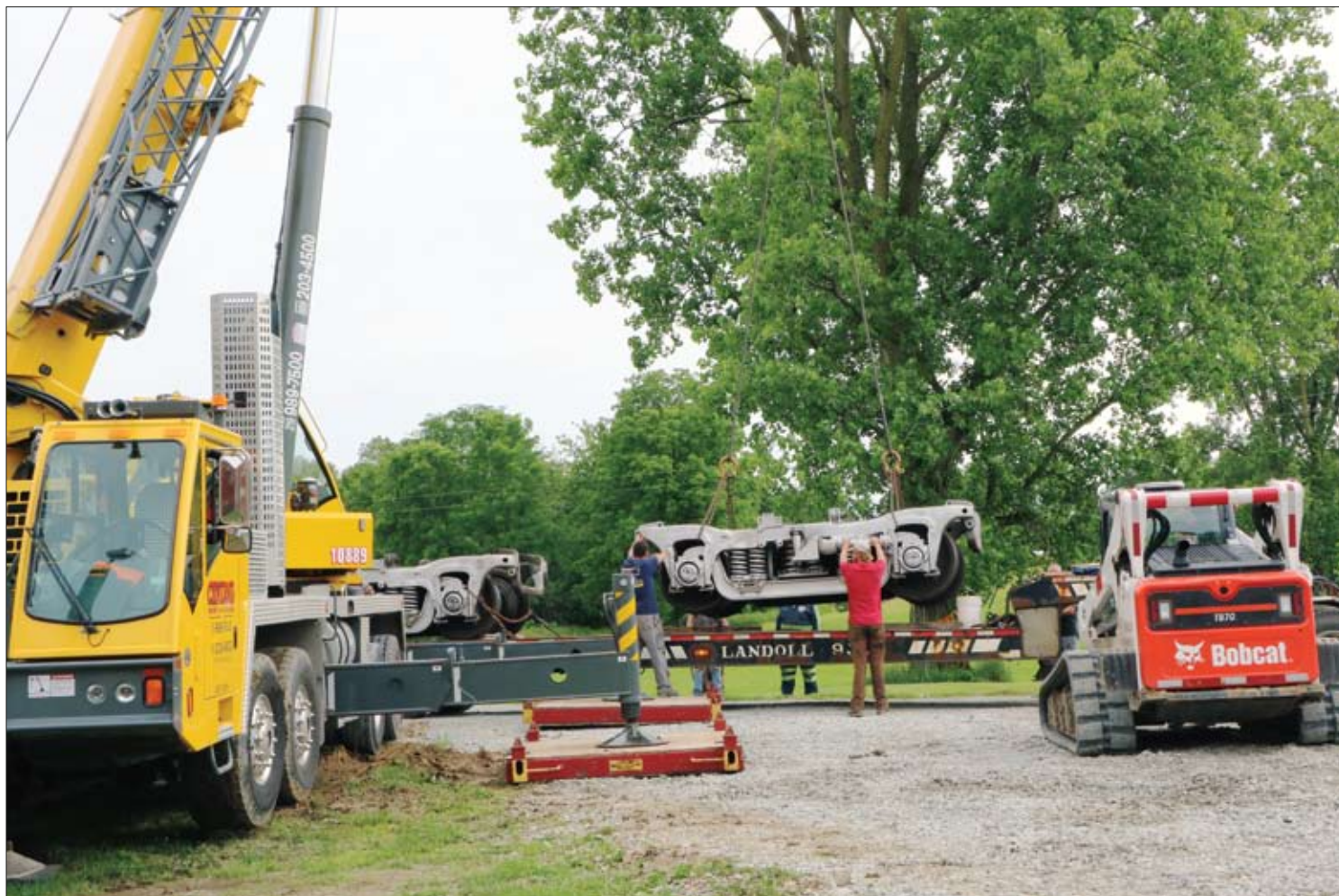
The crane is placing the second set of trucks onto the flatbed trailer for transport to the Miser property.
